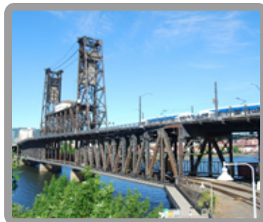
The structurally deficient Steel Bridge in Portland, Oregon, is a critical link for freight rail, passenger rail, light rail, vehicle traffic and those on foot or bike
